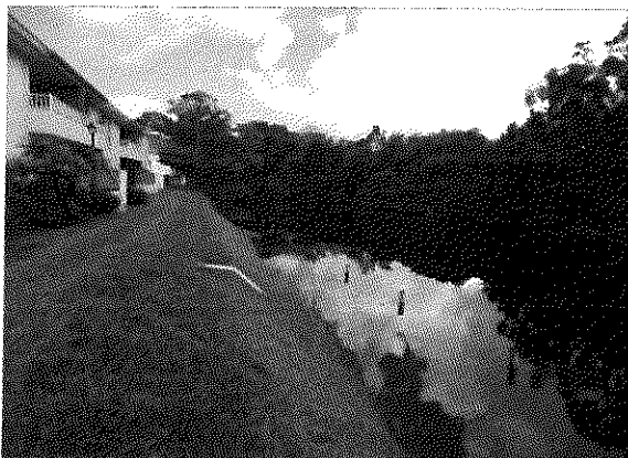
Pond Bank, Note Erosion
