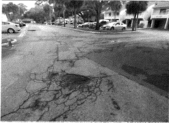
Typical Paving, Note Small Pothole
