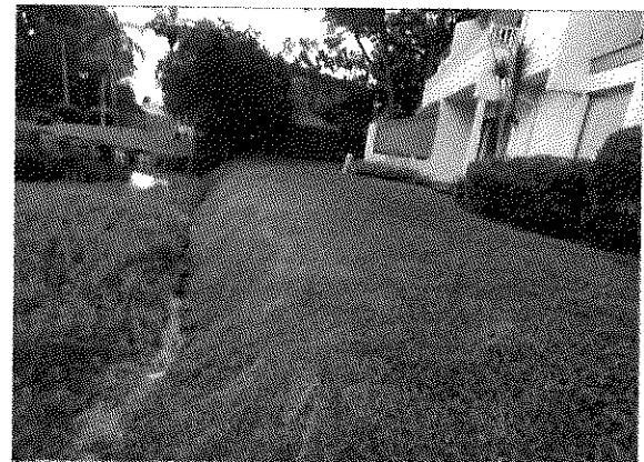
Pond Bank, Note Erosion
